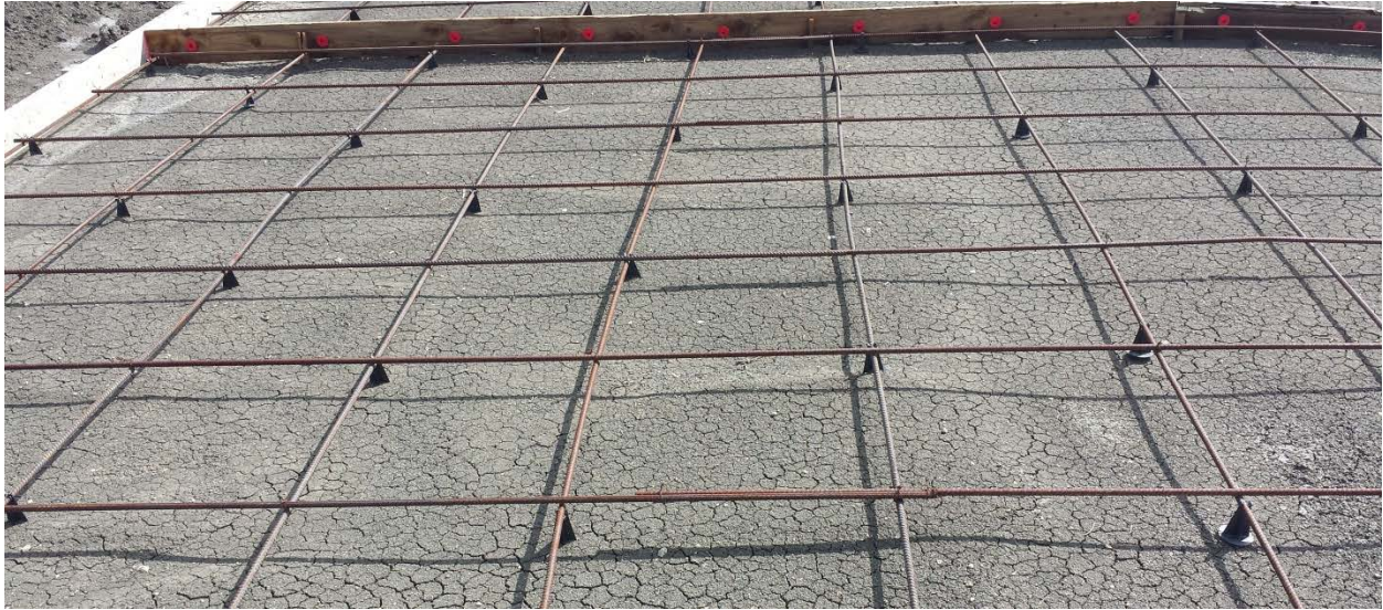
Subgrade is too dry.
