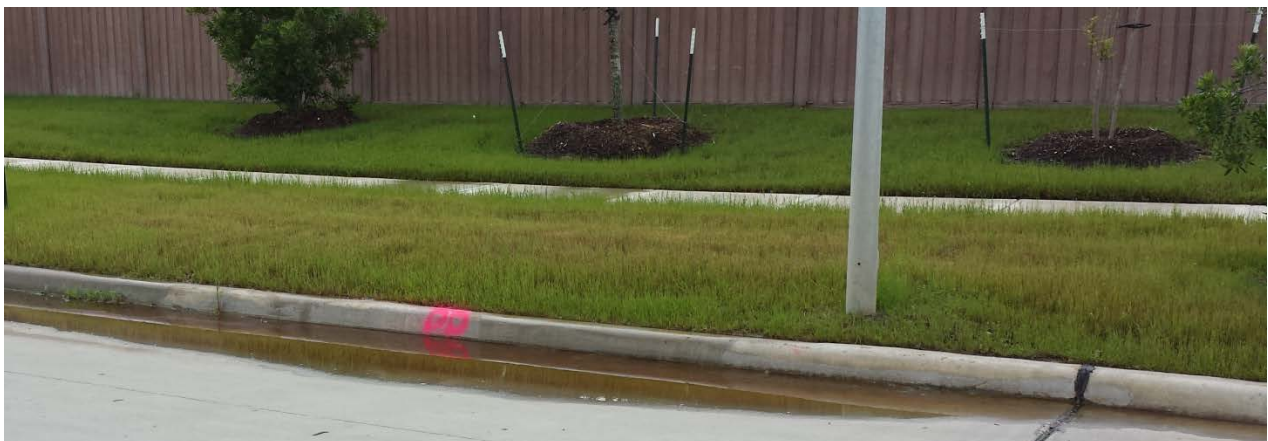
Bird bath has significant length and depth. Lifting, light grinding, or removal of joint sealant obstruction may be acceptable based on field conditions.
