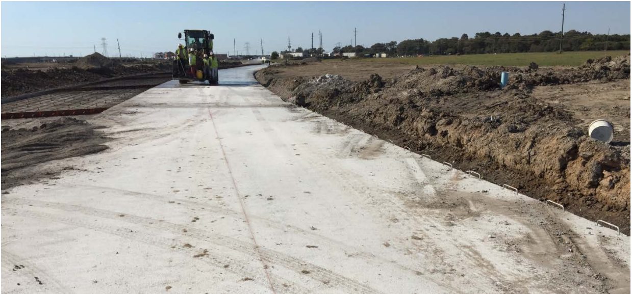
Equipment operating on pavement with inadequate cure time
