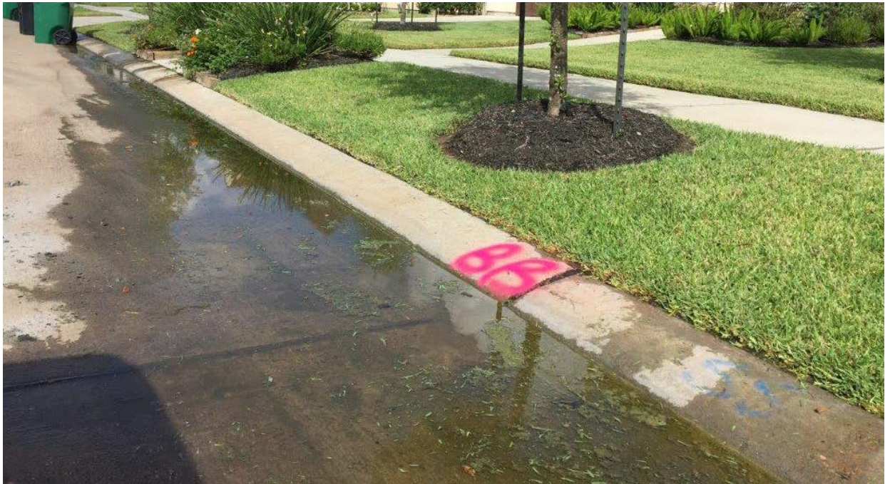
Bird bath extends into driving lane; pavement replacement is required.
