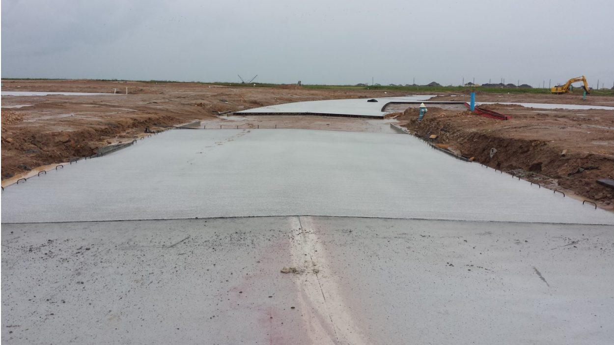
Not saw cutting within specified time (photo shows 4 day old concrete with no sawcuts)
