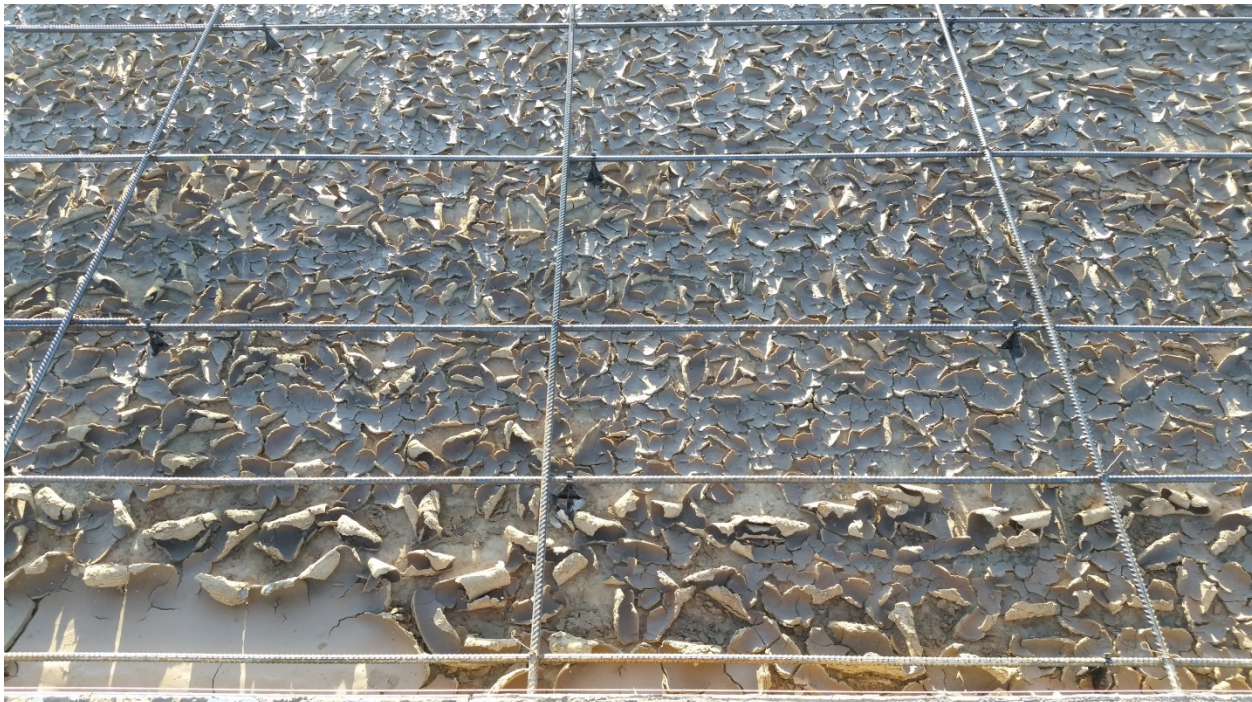
Subgrade is too dry.
