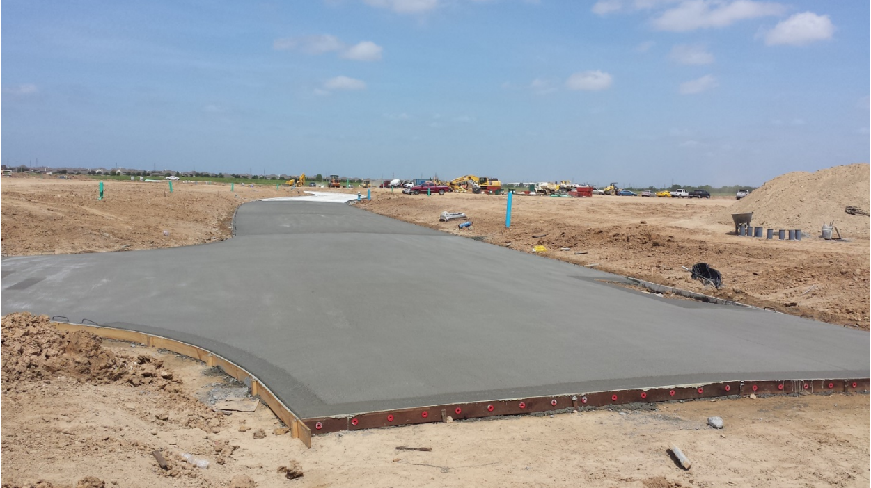
Membrane curing compound not applied to pavement
