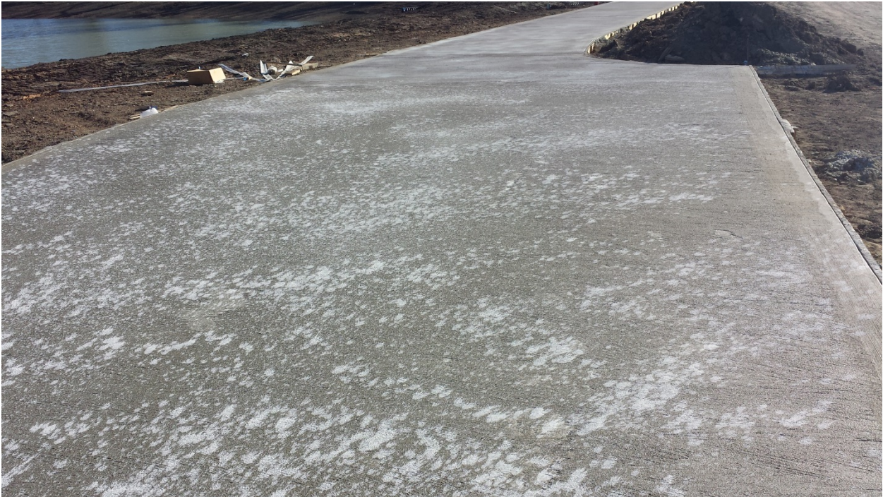
Inadequate curing compound
