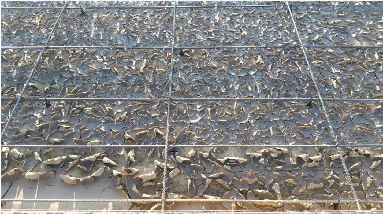
Image 6 - Subgrade is too dry.
