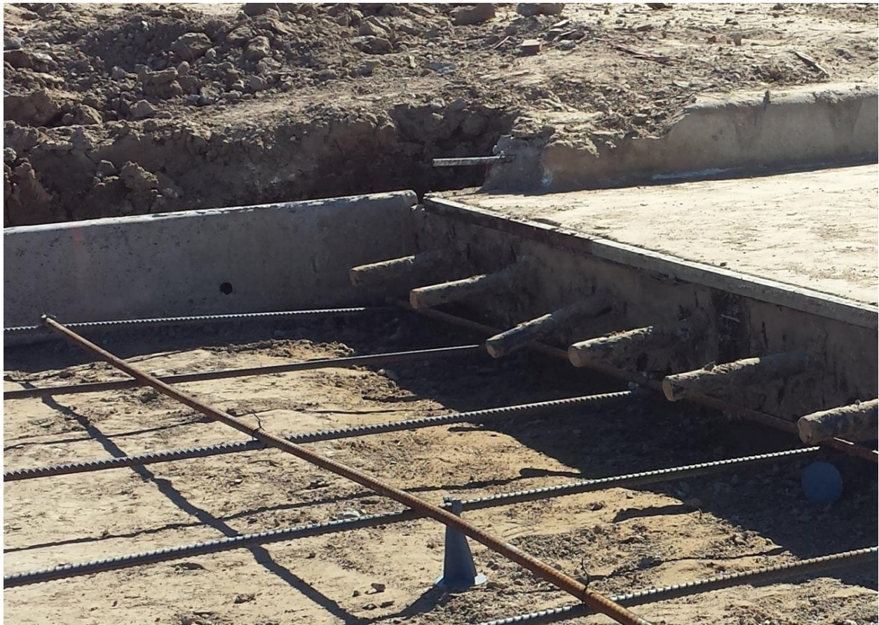
Image 9 - Misaligned dowels may cause spalling near the joint.
