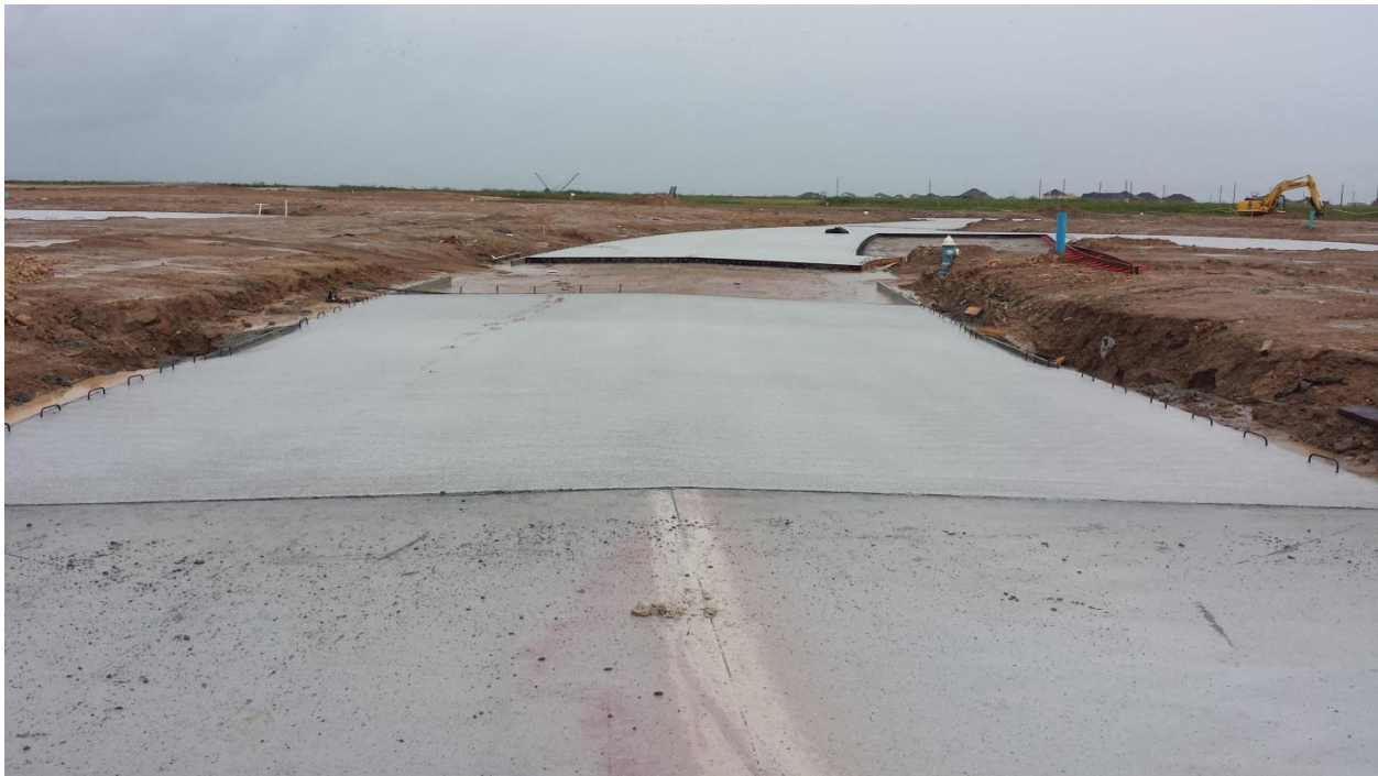
Image 15 - Not saw cutting within specified time (photo shows 4 day old concrete with no sawcuts)
