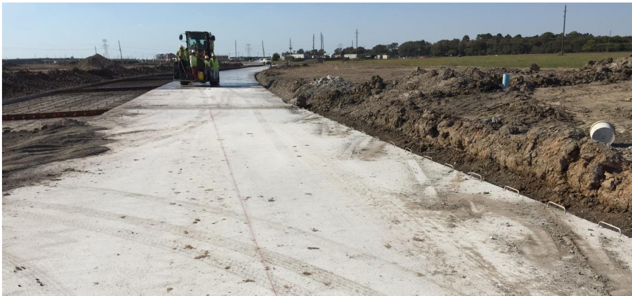
Image 16 - Equipment operating on pavement with inadequate cure time.
