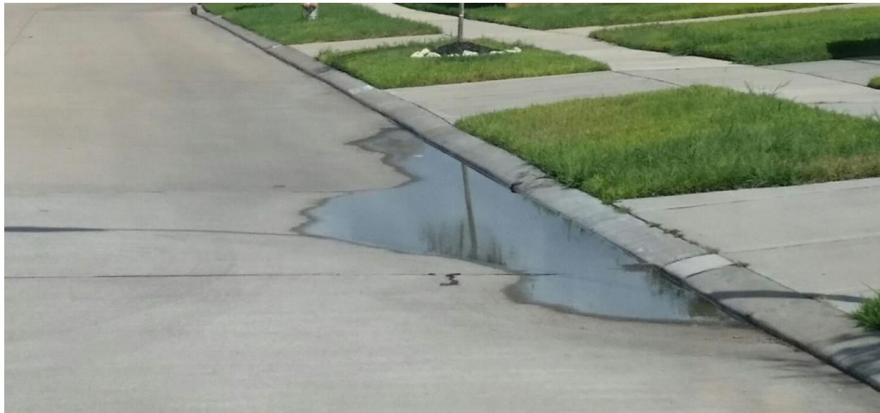
Image 3 - Bird bath has significant length, width, and depth. Lifting or pavement replacement is required. If the lifted pavement cracks then use Concrete Pavement Cracking Evaluation Criteria included in this document.
