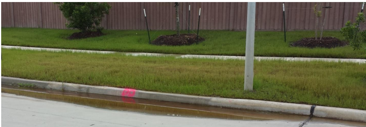
Image 2 - Bird bath has significant length and depth. Lifting, light grinding, or removal of joint sealant obstruction may be acceptable based on field conditions. Grinding shall be limited to 15' either side of the expansion joint.
