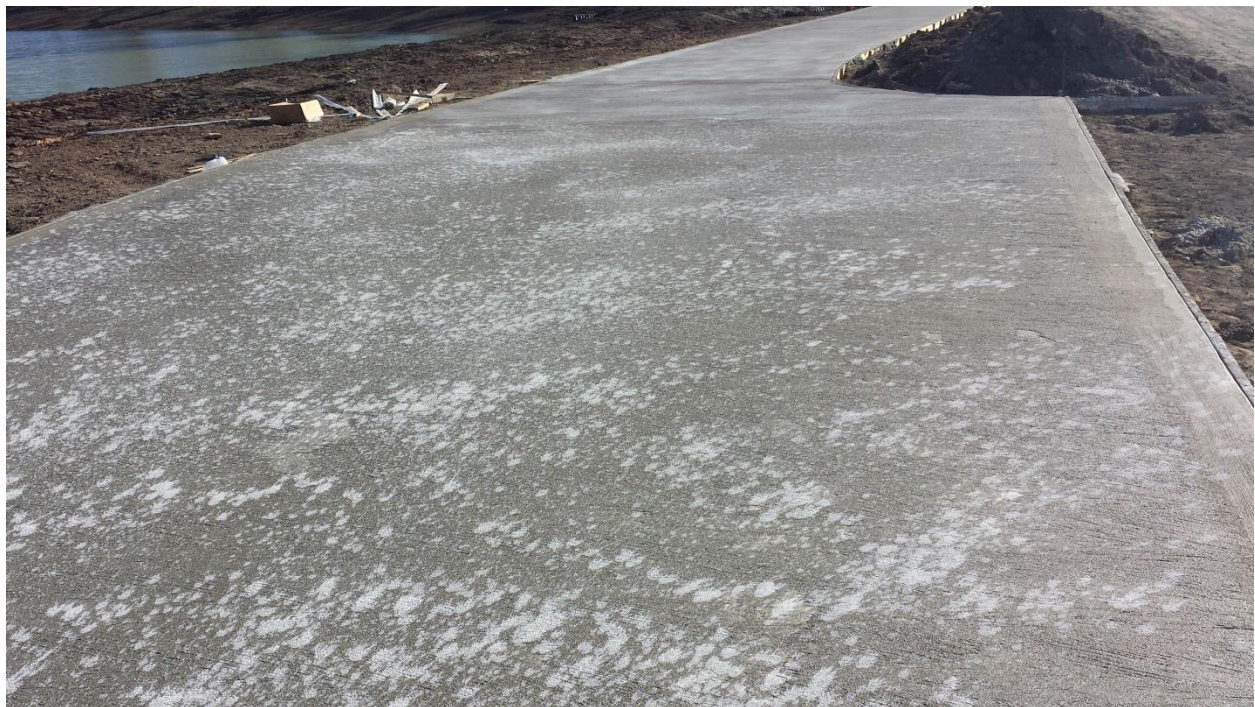
Image 12 - Inadequate curing compound
