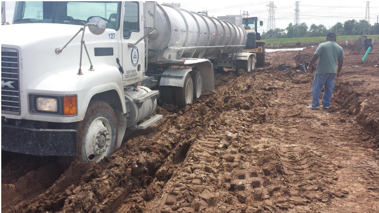
Image 7 - Possible deficiencies in subgrade and base include: Inadequate proof rolling or improper mixing of lime for subgrade, not extending lime mixture to edges of proposed limits of the stabilized subgrade, calculating lime for a 6 inch subgrade and mixing it 8 or more inches deep.
