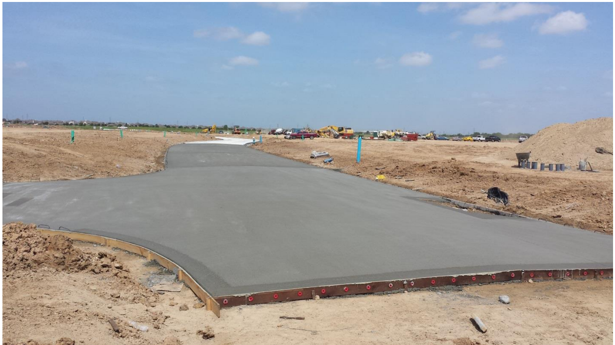
Image 11 - Membrane curing compound not applied to pavement
