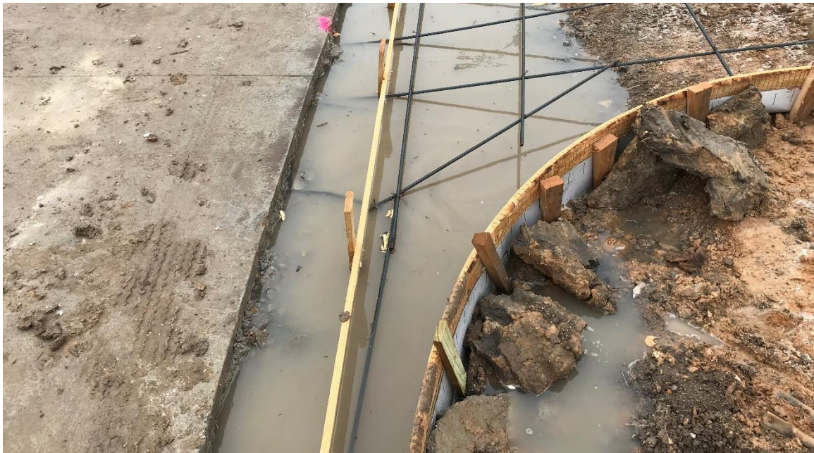
Image 17 - Driveway cut with water sitting weakens the subgrade
