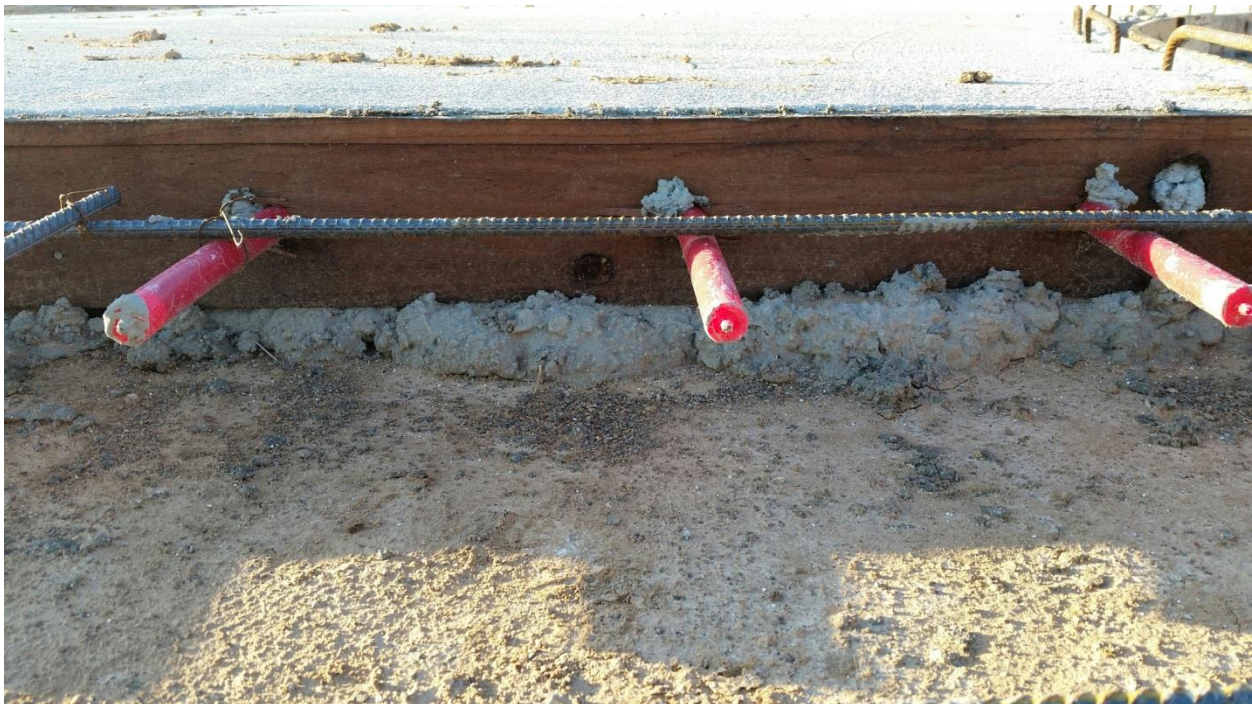
Image 8 - Concrete under headers at expansion joints does not allow expansion to occur correctly.
