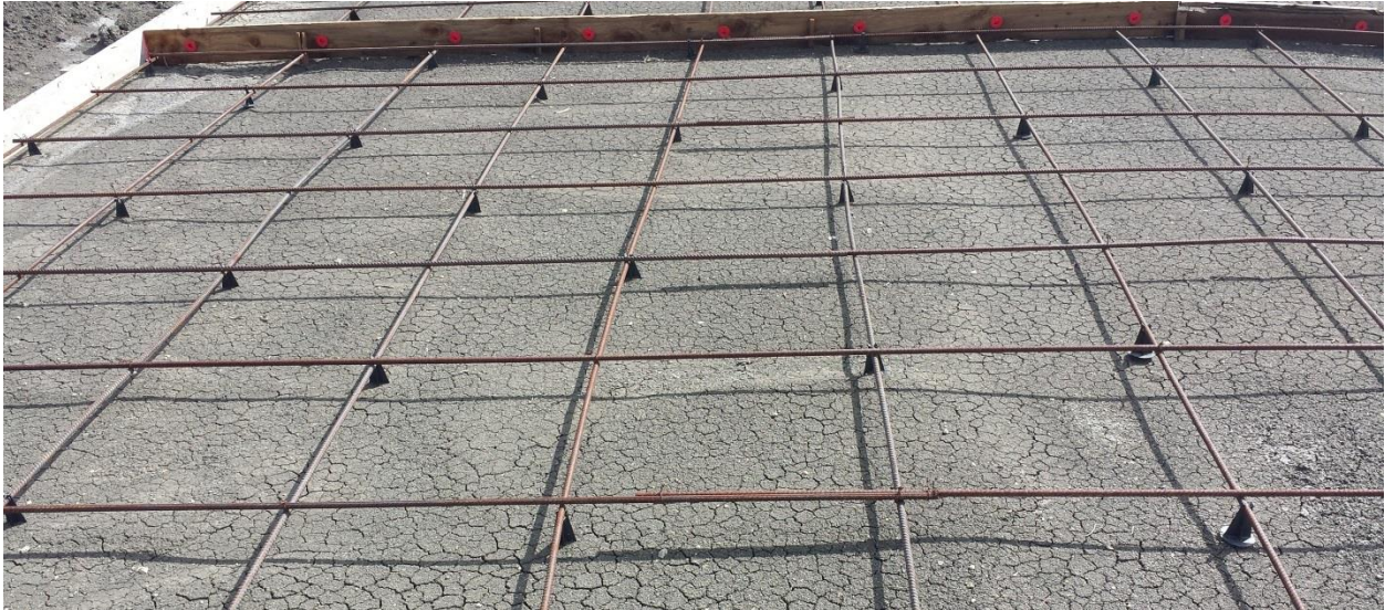
Image 5 - Subgrade is too dry.
