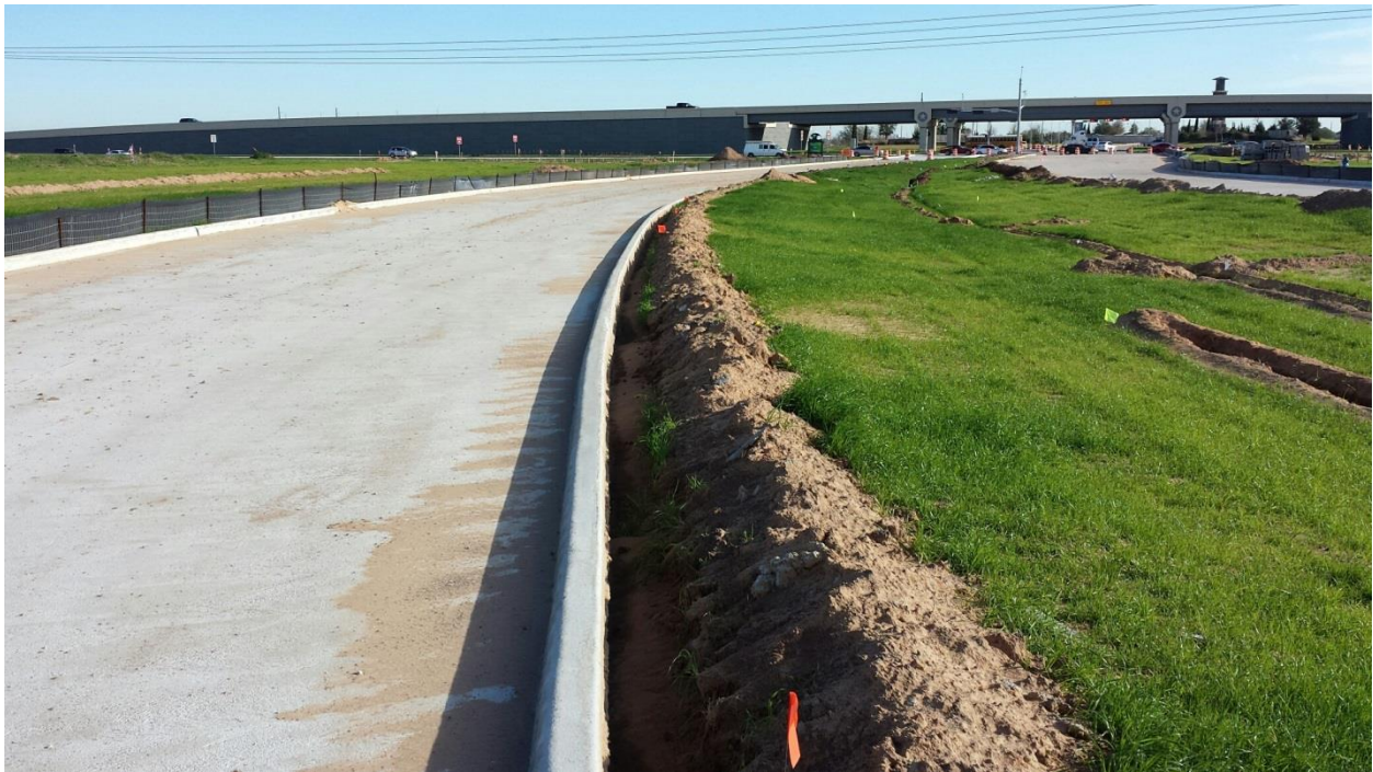
Image 13 - Silt fence or irrigation is placed directly behind curb cuts through subgrade and impacts lateral support.
