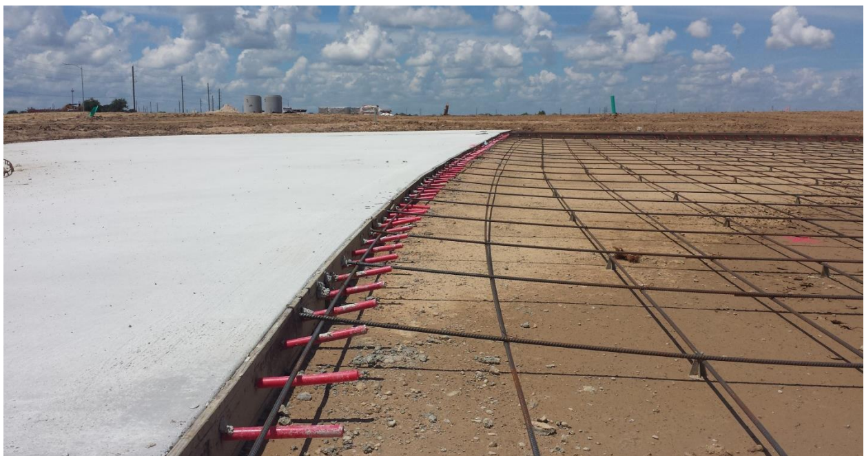
Image 10 - Misaligned dowels may cause spalling near the joint.
