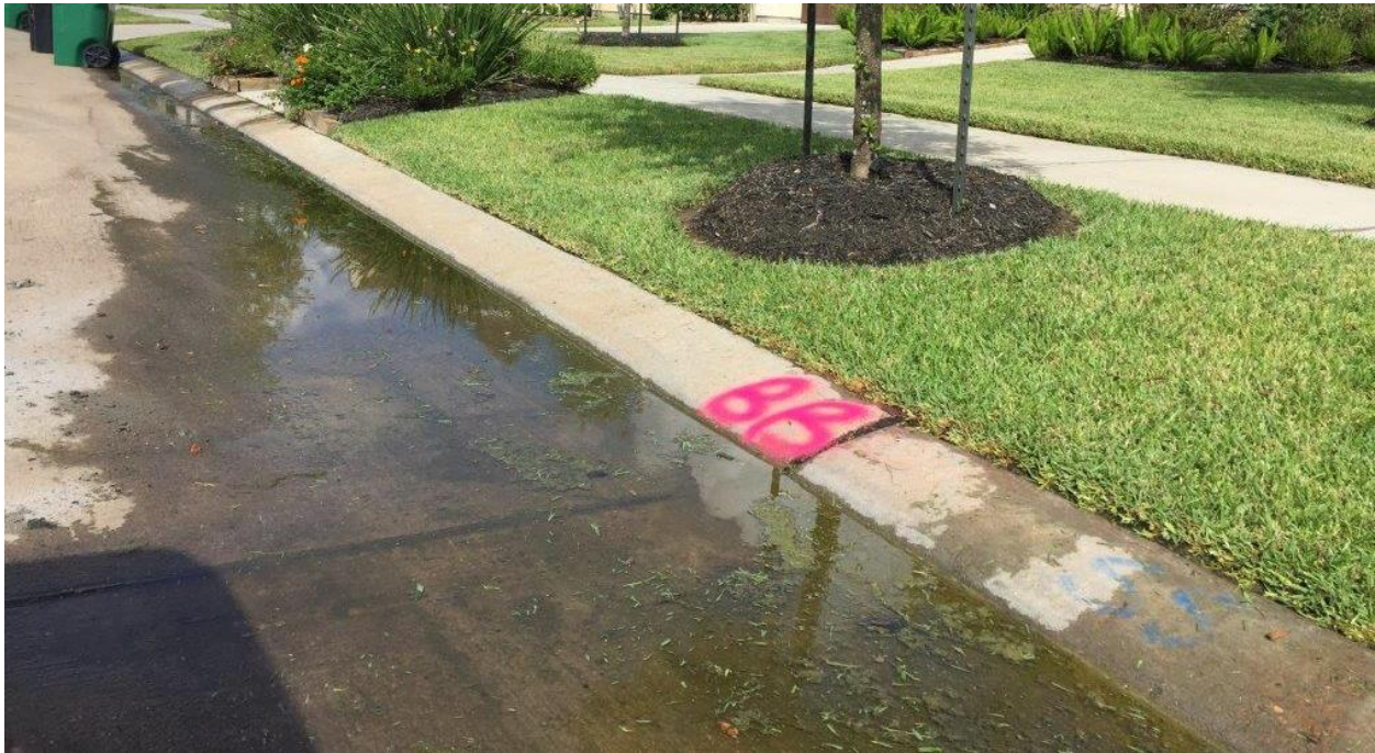
Image 1 - Bird bath extends into driving lane; corrective measures required.
